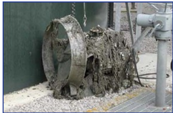
Typical ragged up submersible mixer, which has to be lifted out of the tank for cleaning
